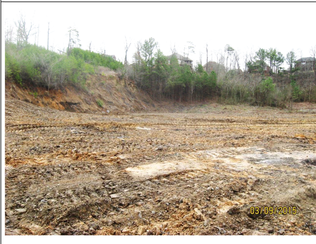
2. A portion of the 4,350 foot Dangerous Highwall after it had been partially backfilled. The average height of this Dangerous Highwall was 50 feet with some areas between 75 and 80 feet.
