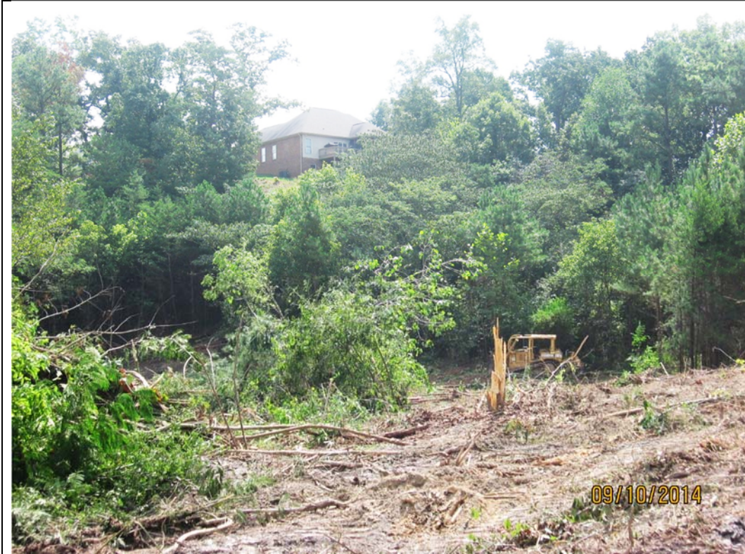
1. Pharris Lane II AML Project in Kimberly, Alabama. This project is adjacent to the Mortimer Jordan High School Athletic Complex.
