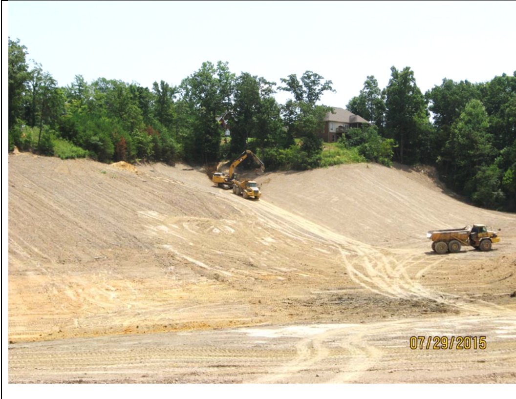
3. This portion of the Dangerous Highwall was adjacent to a subdivision and at one point was within 75 feet of a couple of houses.
